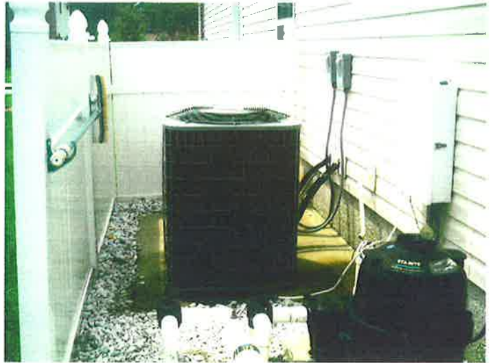
CONDENSING UNITS & PLATFORM 07/28/2010
