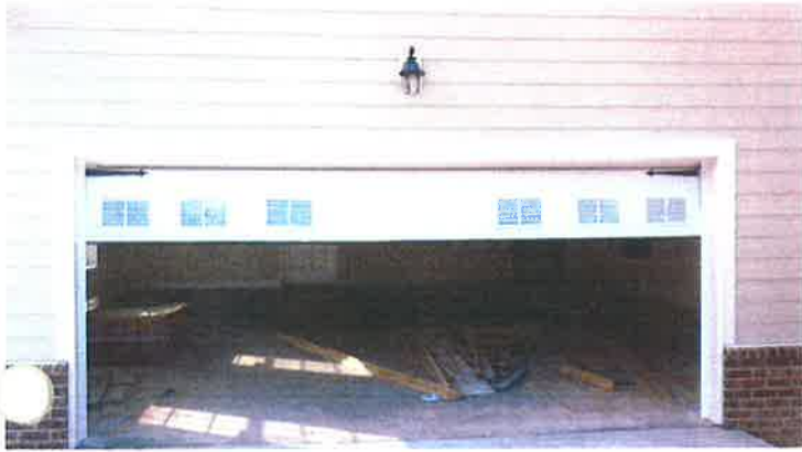
GARAGE DOOR FLOOD VENTS 08/26/2010
