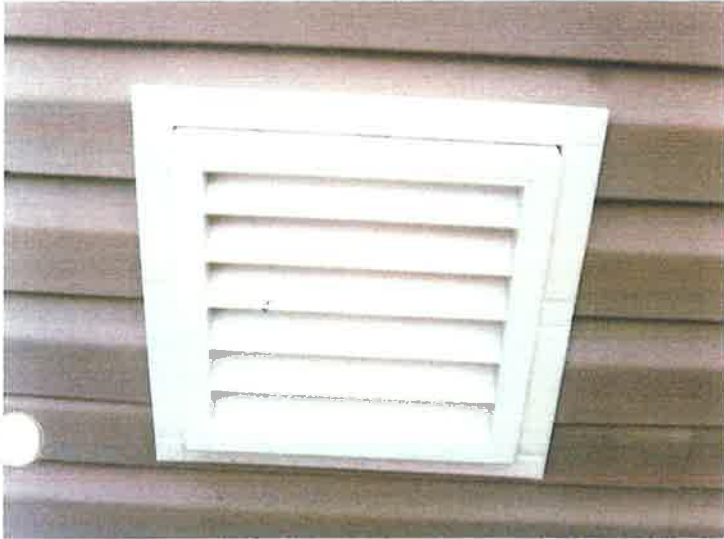
TYPICAL VENT (GABLE VENT) USED IN GARAGE WALL 05/03/2010
