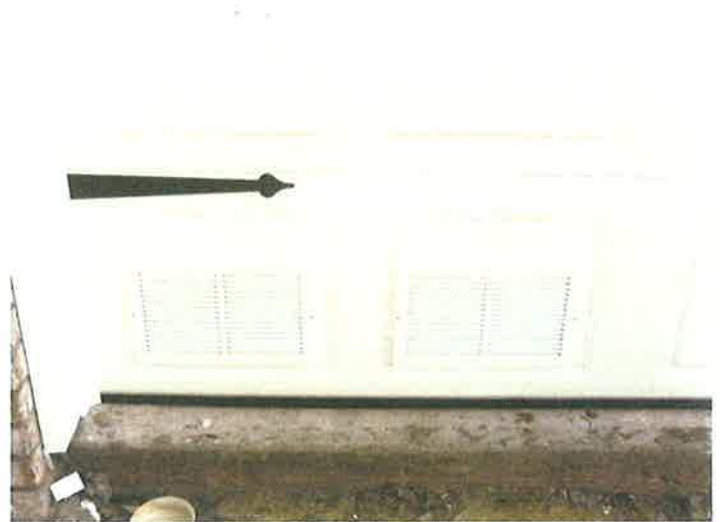
TYPICAL VENT USED IN GARAGE DOOR 05/03/2010
