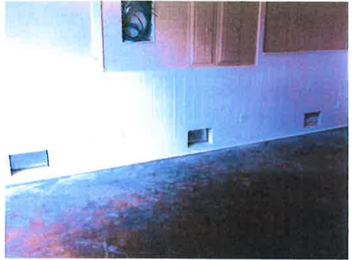
INTERIOR VIEW OF SMART VENT FLOOD VENTS LOCATED IN GARAGE/MODEL HOME OFFICE 3/26/2013
