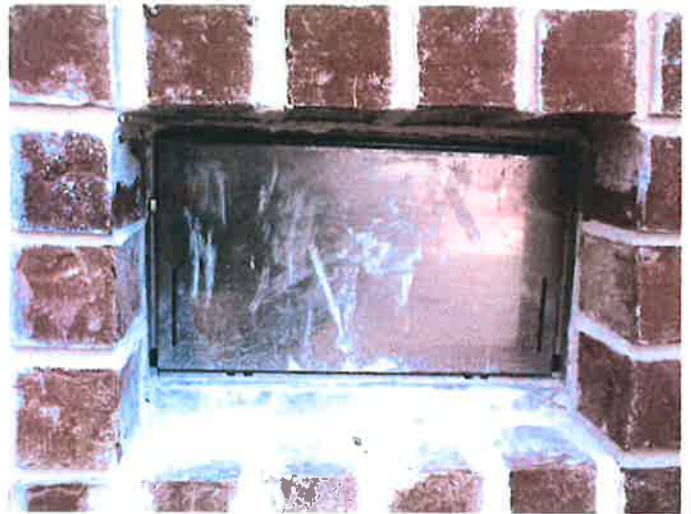
TYPICAL SMART VENT FLOOD VENT 3/26/2013
