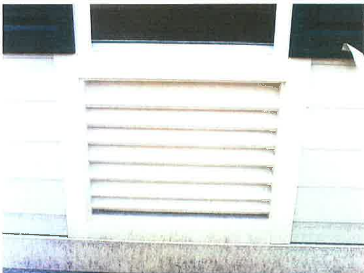
VENT IN ENCLOSURE(GARAGE) WALL (TYP) 06/08/2010
