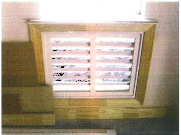
VENT IN ENCLOSURE(GARAGE) WALL (TYP) 06/08/2010
