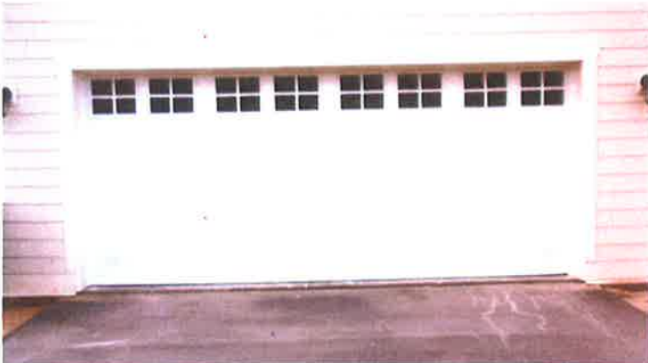
VENTS IN GARAGE DOOR 06/30/2011
