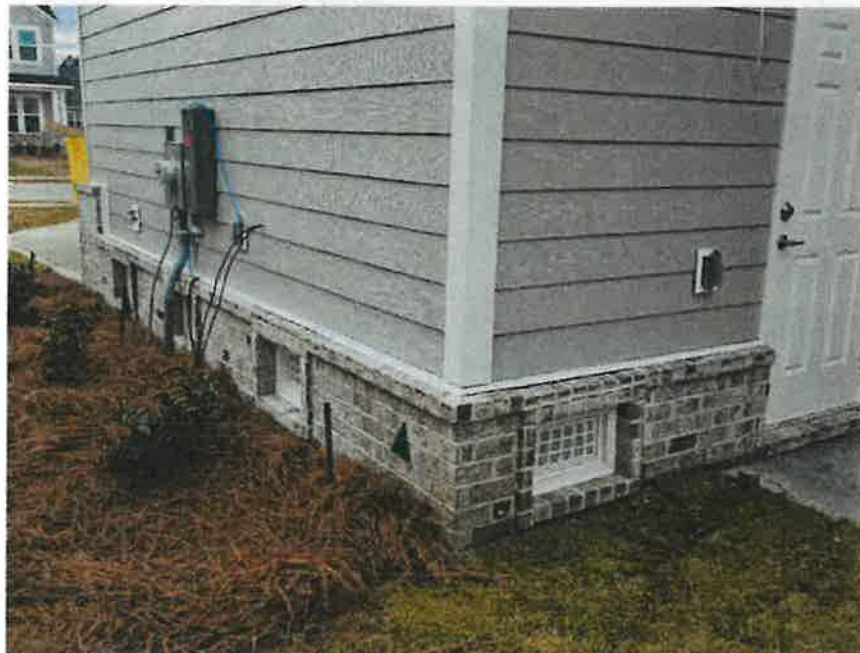
Photo Two Caption Vent Pic 2 2/24/25
